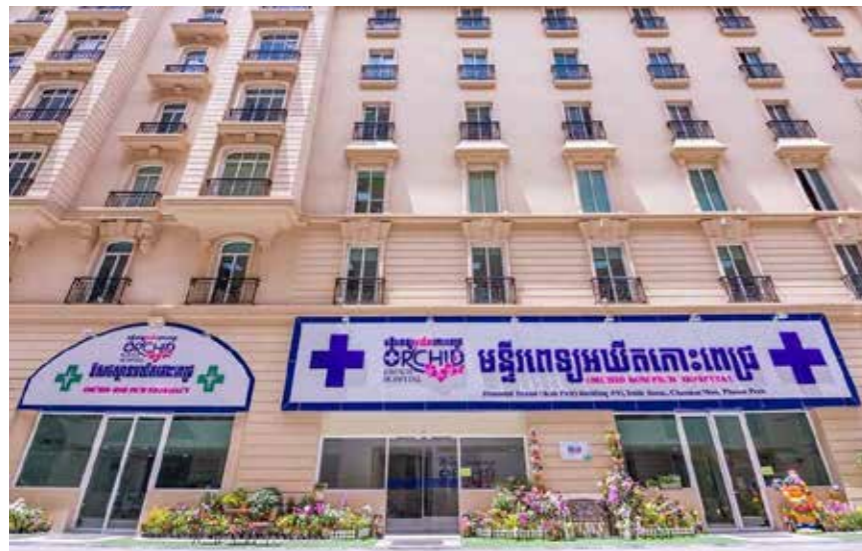
Orchid Kohpich Hospital Design&Build (Structural Strengthening& Interior Decoration,MEP) Building Area: 408m2 Total Floor area:3672m2
